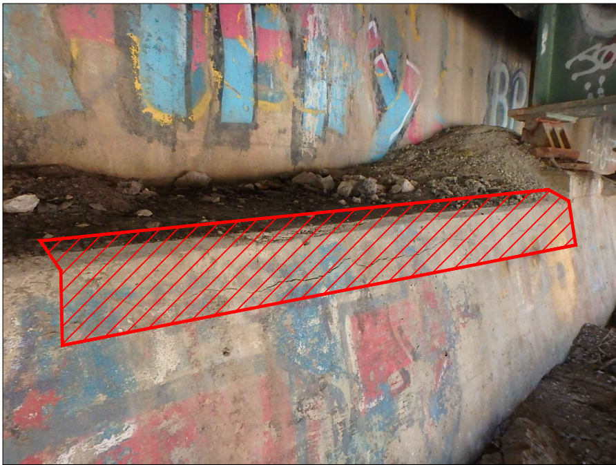
CRACKED AND DELAMINATED WEST ABUTMENT FOOTING
