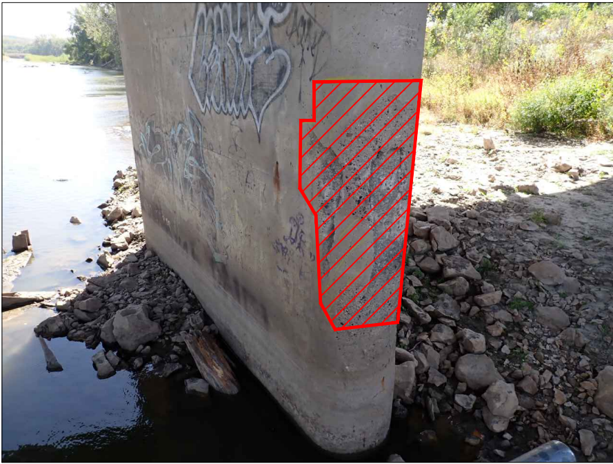
SPALLED PIER #1 STEM AT NORTH END
