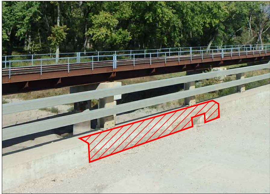
TYPICAL DELAMINATED CURB
