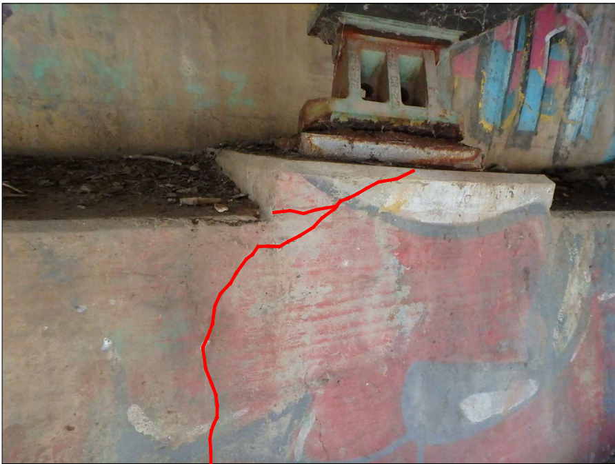
CRACKED WEST ABUTMENT FOOTING
